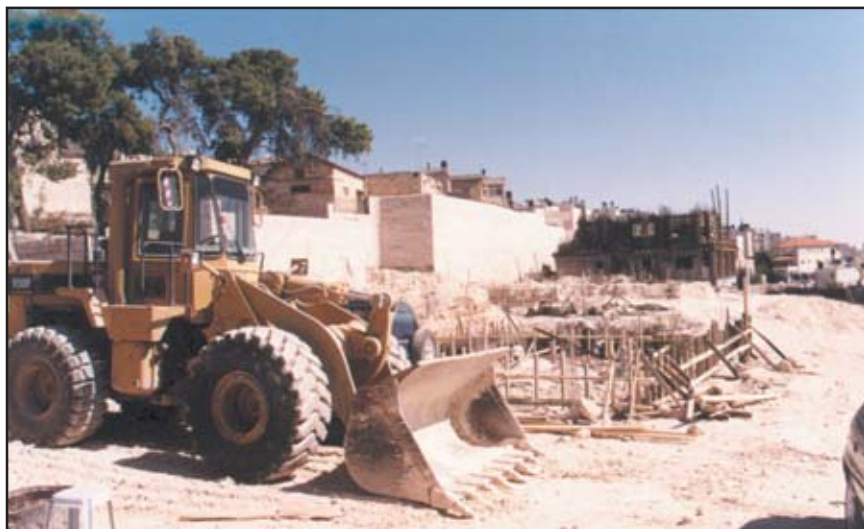
(Above) New construction of the housing project over the last several months.
